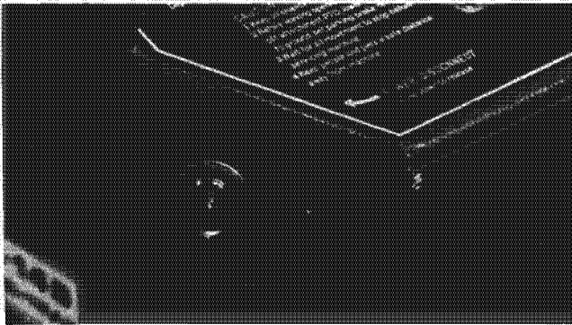
FIG. 1. Tractor Power Disconnect Switch
